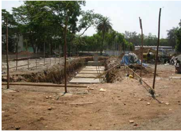
Indoor Stadium balance foundation work in progress {Actual work photograph taken on March 15, 2008}
