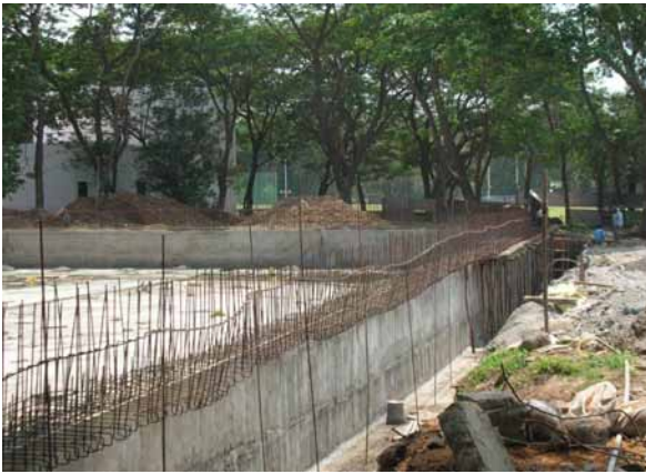
Swimming Pool overflow channel work in progress {Actual work photograph taken on March 15, 2008}
