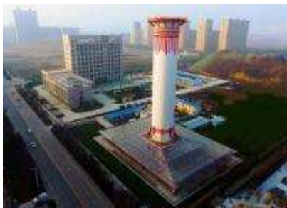
Filters installed in smog tower, IIT Bombay team begins to study
