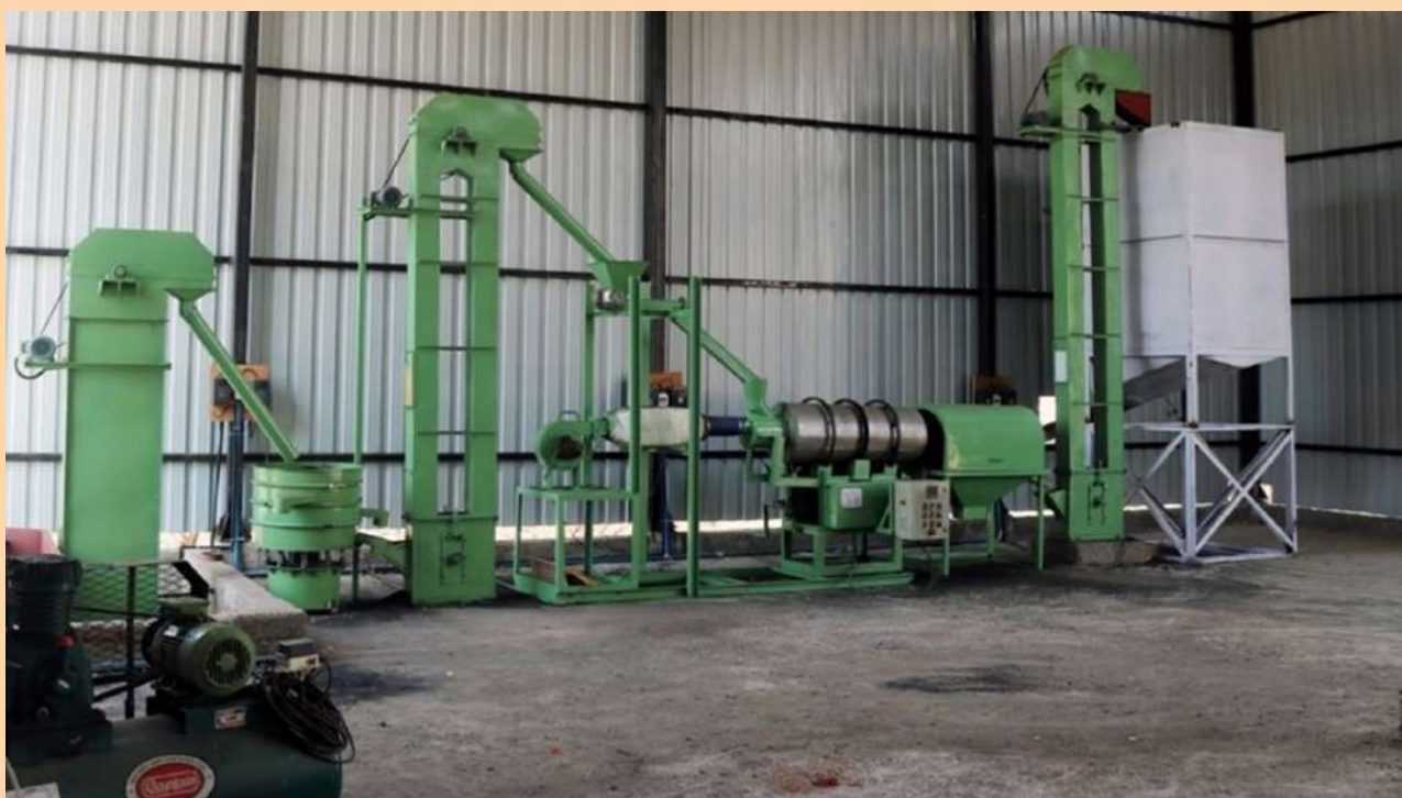
Plant for sand reclamation based on IITB Technology- transferred to Deccan Crest Pvt Ltd.
