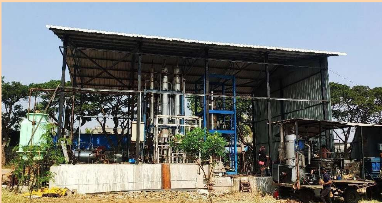
The mobile and stationery jaggery powder plants based on IITB technology installed in Kolhapur
